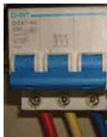
Picture 10 Air Switch
